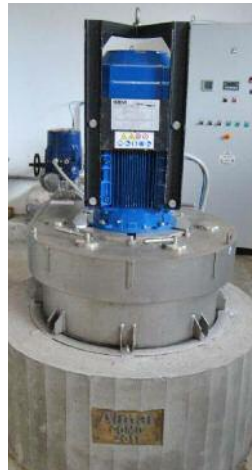
On the left, the new microturbine
